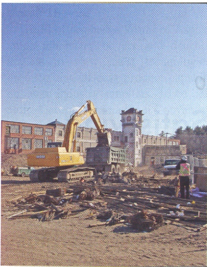
With Clocktower building earmarked for renovation in background, Catalano Construction's John Deere excavator loads demolition debris on a Mack truck.
