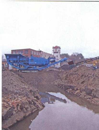
Shattered boulders and demolition debris are pulverized by mobile Terex/Pegson crusher for reuse on-site. (D. Joubert photo)
