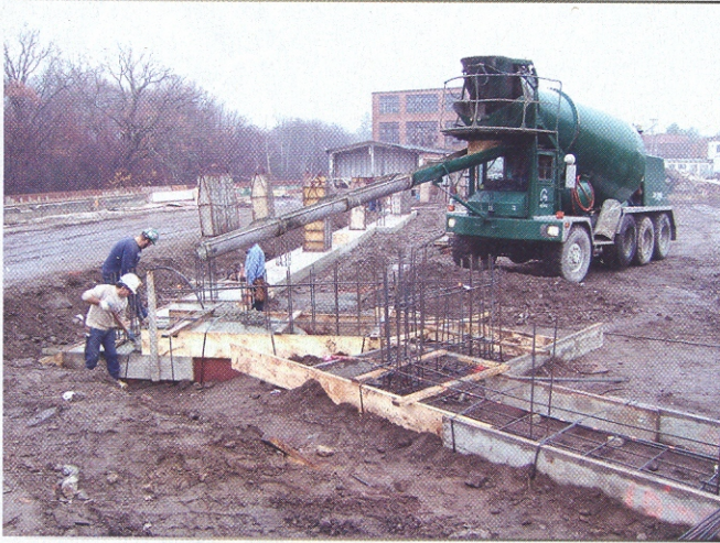
Greenville Ready Mix truck supplies concrete to workers as they place spread footings. (D. Joubert photo)
