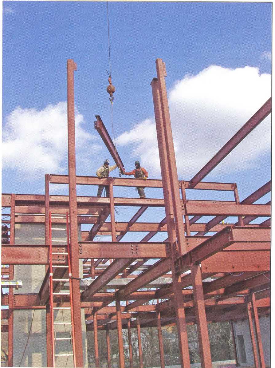
Ironworkers set beam for new Burrillville, R.I., library under construction by E.W. Burman.
